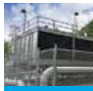
Cooling Water Treatment
